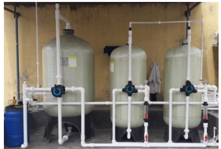
IRON REMOVAL SYSTEMS
