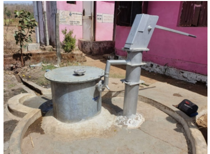
FLUORIDE REMOVAL SYSTEMS
