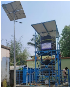
SOLAR POWERED IRON / ARSENIC / FLUORIDE UNIT SYSTEM
